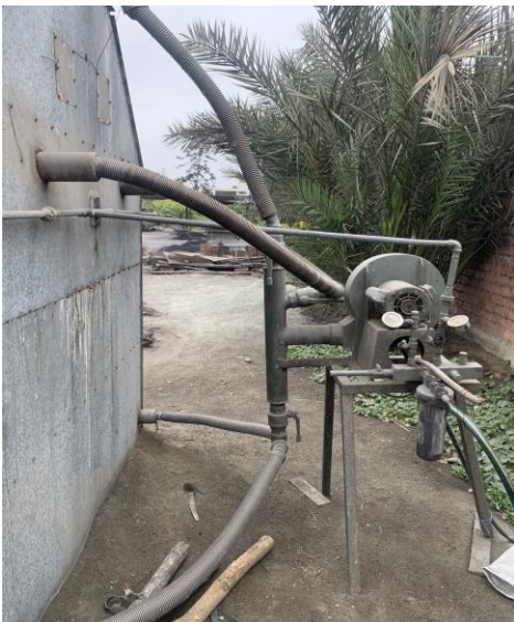
Auxiliar equipment: water pump
