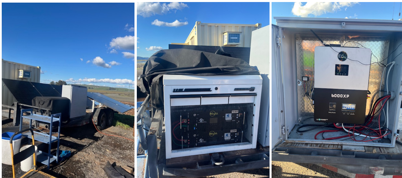
Figure A2-4. Solar array (left), Battery storage (center) and energy meter (right)
